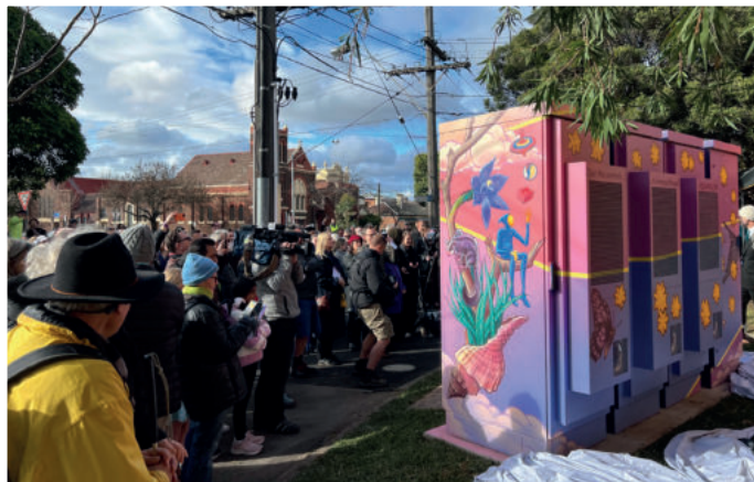
Neighborhood battery in Victoria, Australia
