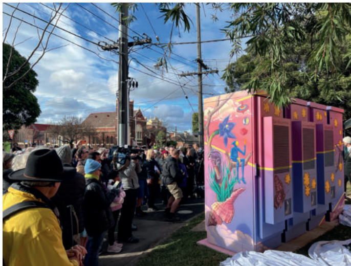
Neighborhood battery in Victoria, Australia
