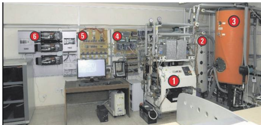
Figure 4. Experimental trigeneration installation with system of integration of additional energy sources based on RES
