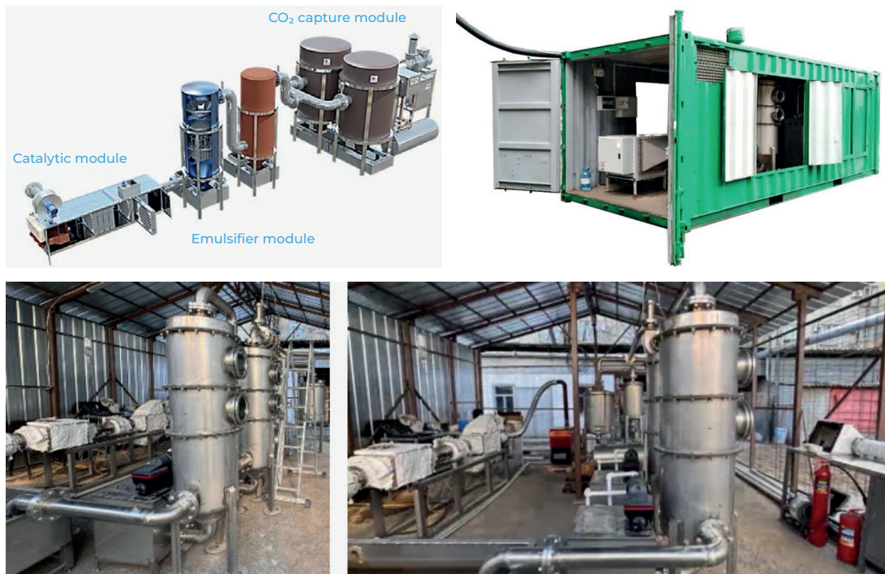
Figure 1. Integrated Cleaning System
