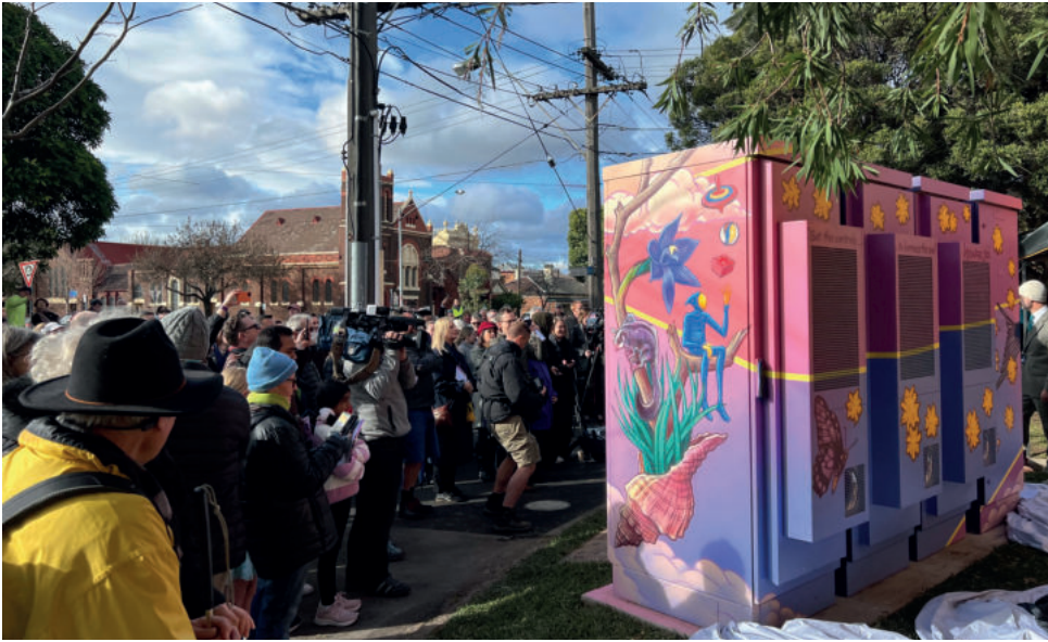
Neighborhood battery in Victoria, Australia
