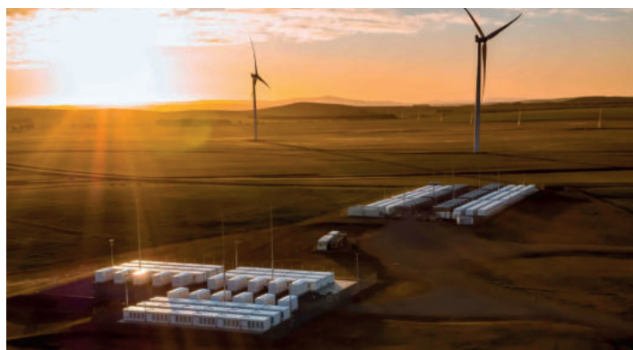
Hornsdale Power Reserve and Hornsdale Wind Farm
