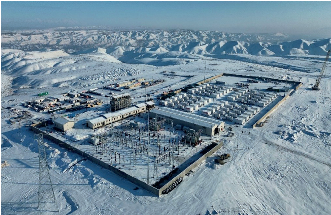
The Lochin 150MW/300MWh energy storage project
